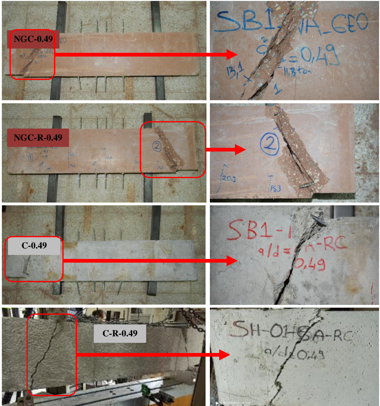
Figure 3-58 Close look-up to the final state of shear cracks of test specimens with an a/d ratio of 0.49
