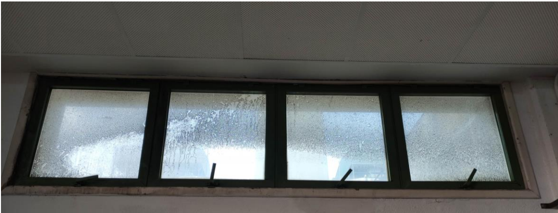
Figure 78. Small windows of the building
