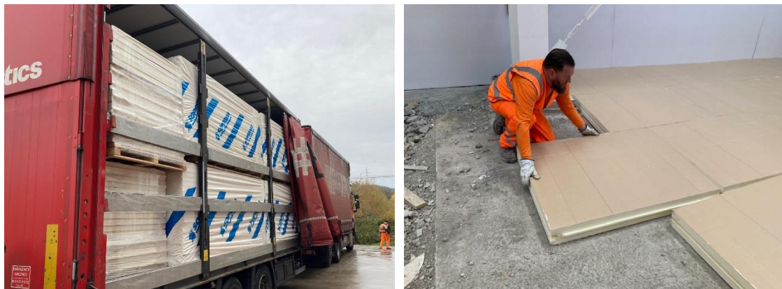
Figure 87. Reception on site of insulating material sent by SOPREMA and test installation on the ground.
