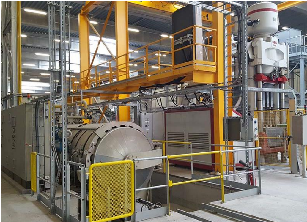
Figure 54. Orbix carbonation pilot facilities.
