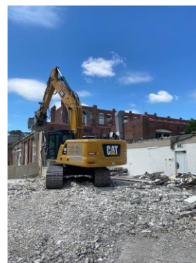
Figure 14. Demolition crane on site (photographed by Frank Rens and Bente Kamp, GBN)
