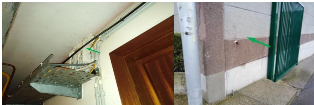
Figure 51. Two applications tested for asbestos (left: coating, right: putty between concrete panels).
