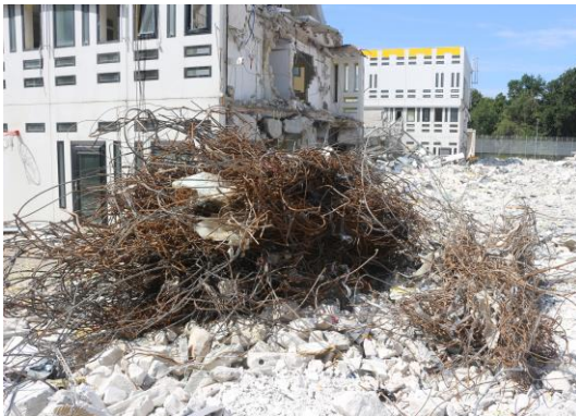
Figure 17. Removal of iron rebar (photographed by Frank Rens and Bente Kamp, GBN)
