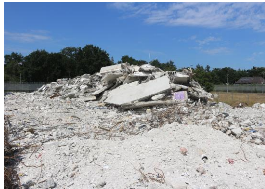
Figure 18. Clean concrete before it was reduced in size to make it small enough for crushing
