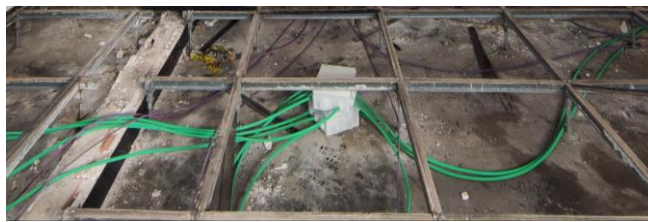
Figure 82. Wires in the building.
