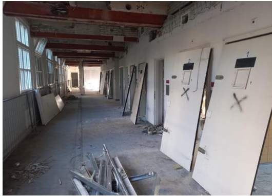
Figure 11. Stripped area, collection of doors and cable trays (photographed by Frank Rens and Bente Kamp, GBN)
